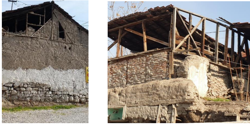
Figure 3.5: Structural system details from the houses at Dutlu and Sarıkadı Streets (Çakıroğlu, 2021)
