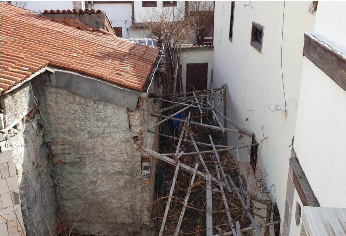
Figure 3.47: An example to the use of incompatible materials for the repair of old buildings at Hamamönü (Çakıroğlu, 2021)
