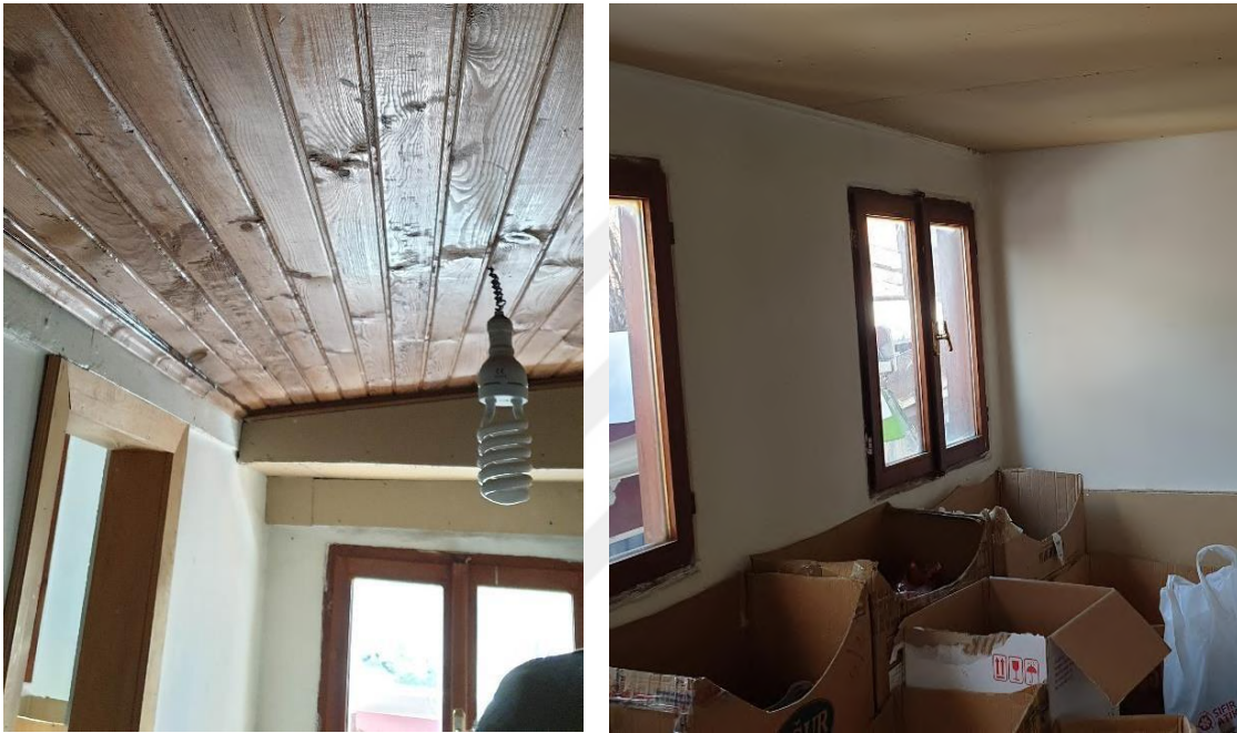
Figure 3.32: Inappropriate usage of the rooms on Dutlu Street (Çakıroğlu, 2021)
