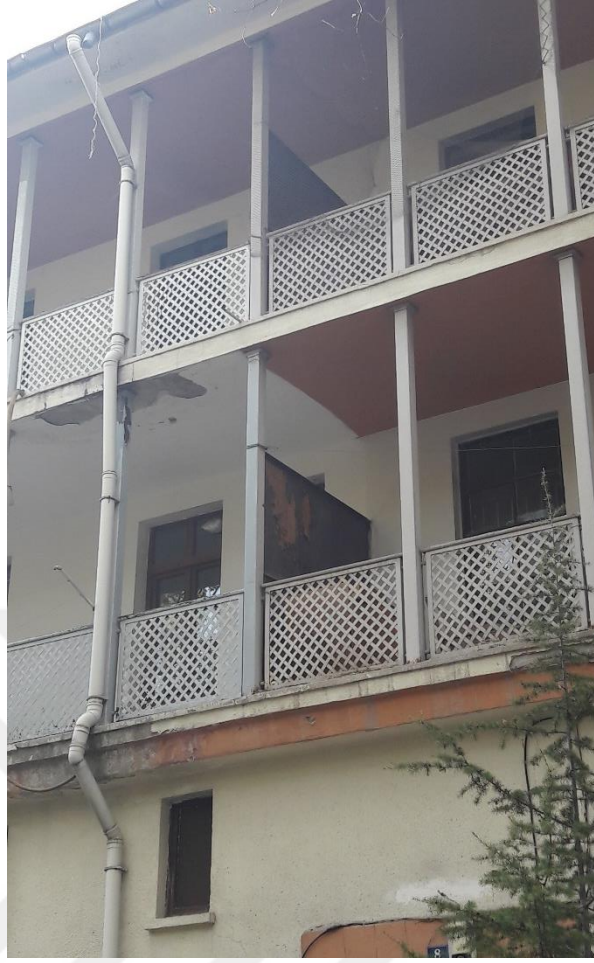
Figure 4.2: Decay on the building facades (Başagaç, 2017).
