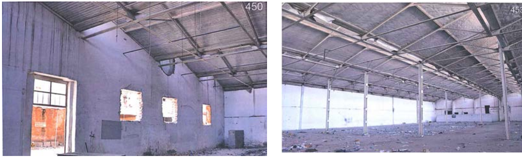
Figure 4.77: Inside the Structures of Yarn Building ( 2014, Adana Directorate of Surveying Monuments Archive by Miyar Architecture)
