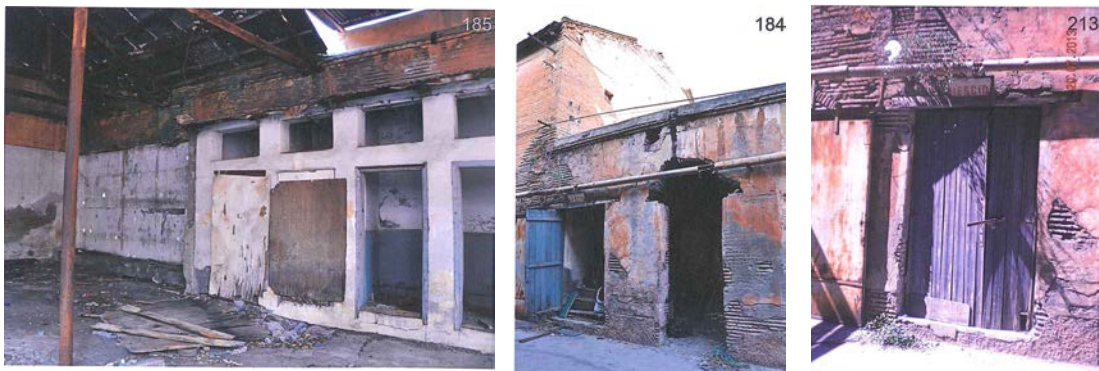
Figure 4.55: The Old Factory's Wet Volumes ( 2013, Adana Directorate of Surveying Monuments archive by Miyar Architecture)
