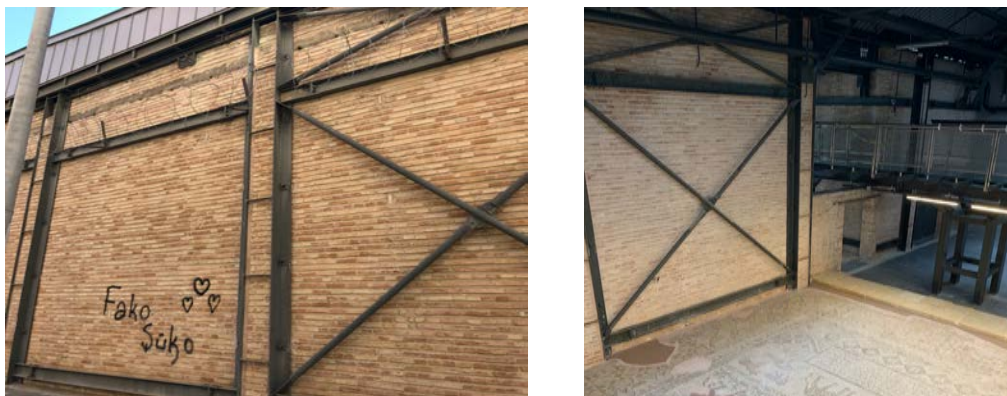
Figure 4.46: The Old Brick Wall With Steel Supporters Outside and Inside of Adana Museum Complex (2019, Çağlayan, S.)
