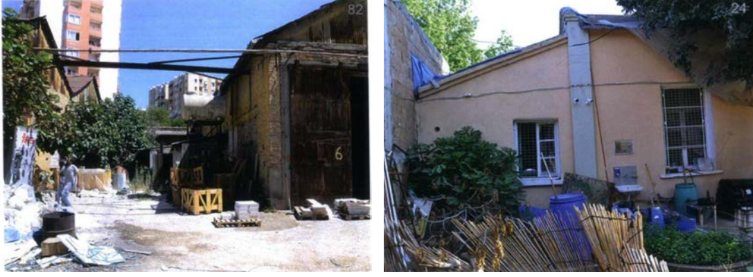
Figure 4.39: Small Toilet and Infarmacy (2013, Adana Directorate of Surveying Monuments archive by Miyar Architecture)
