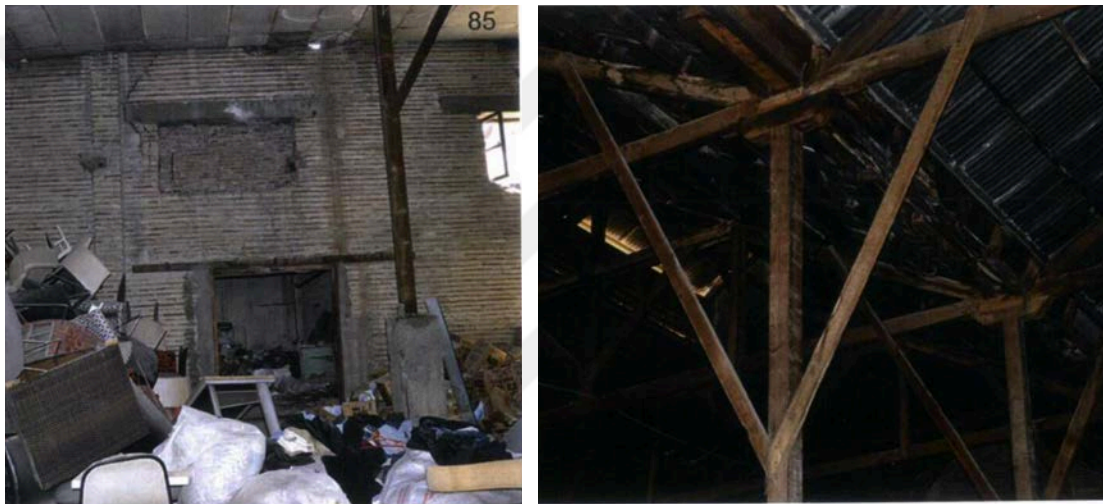
Figure 4.37: Concrete Beams and Wooden Posts (2013, Adana Directorate of Surveying Monuments Archive by Miyar Architecture)
