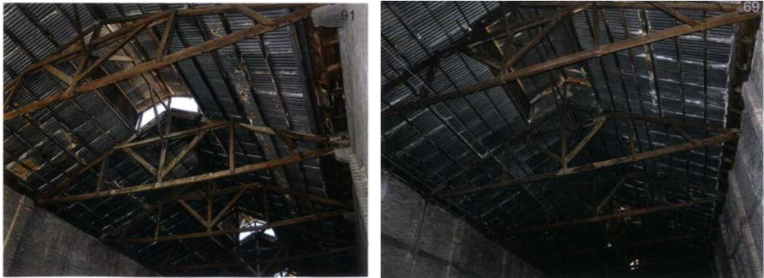
Figure 4.36: Roof Openings of Warehouses (2013, Adana Directorate of Surveying Monuments archive by Miyar Architecture)
