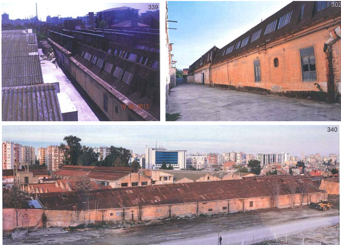
Figure 4.69: Exterior of Weaving Building (2014, Adana Directorate of Surveying Monuments Archive by Miyar Architecture )
